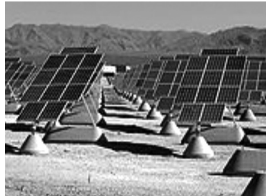
Fig. 4. Photovoltaic panels of a solar power plant [6]
