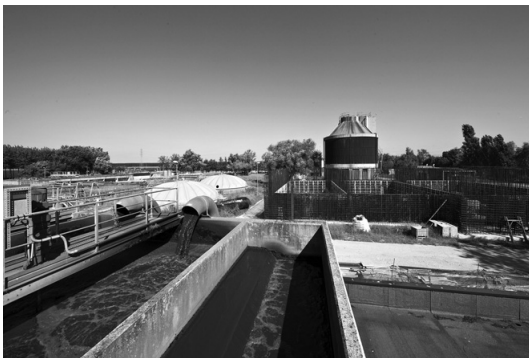
Fig. 2-3. Details of Water pumping Mt. Calvario Gorizia station and Waste water treatment plant of Bistrigna (Staranzano) (Source: Irisacqua Ltd)
